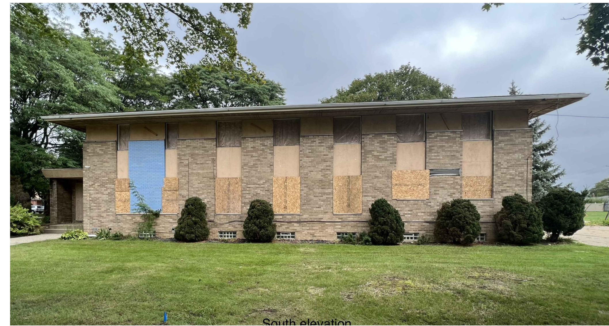
1A DEMOLITION ELEVATION AD1.0 SCALE: NOT TO SCALE PHOTO ISSUED FOR REFERENCE ONLY
