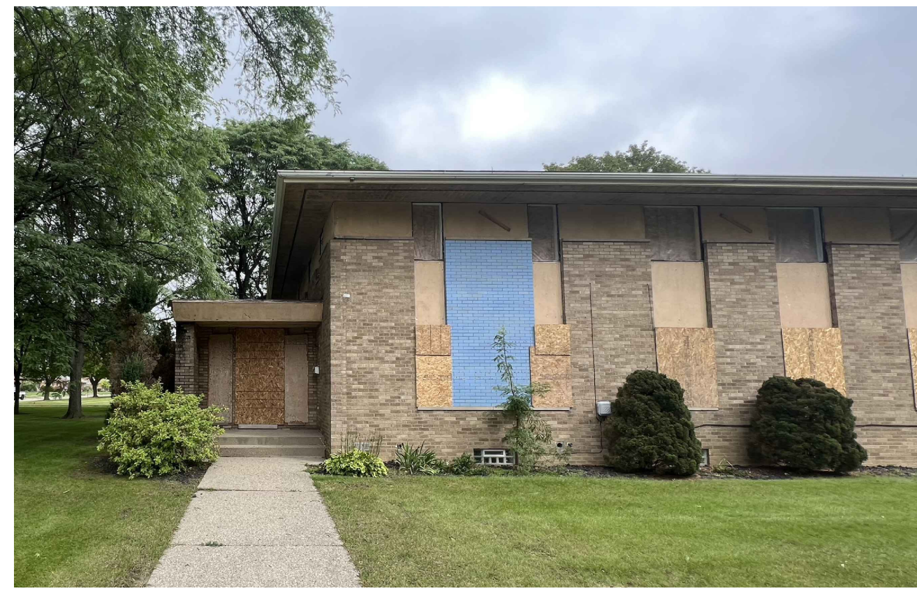
1B DEMOLITION ELEVATION AD1.0 SCALE: NOT TO SCALE PHOTO ISSUED FOR REFERENCE ONLY
